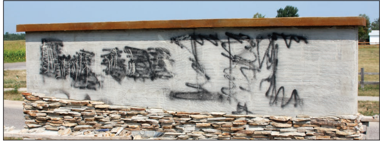
Before: Graffiti covered the welcome sign along the Moccasin Road entrance.
